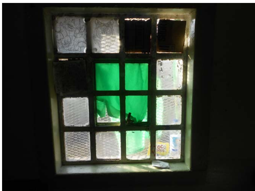
Figure 5: Cardboard replacing glass panels on C wing at HMP Swinfen Hall (inspected in October 2016)
